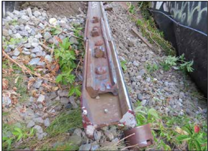
Figure 3. Ruptured rail on the CC Long Siding track
